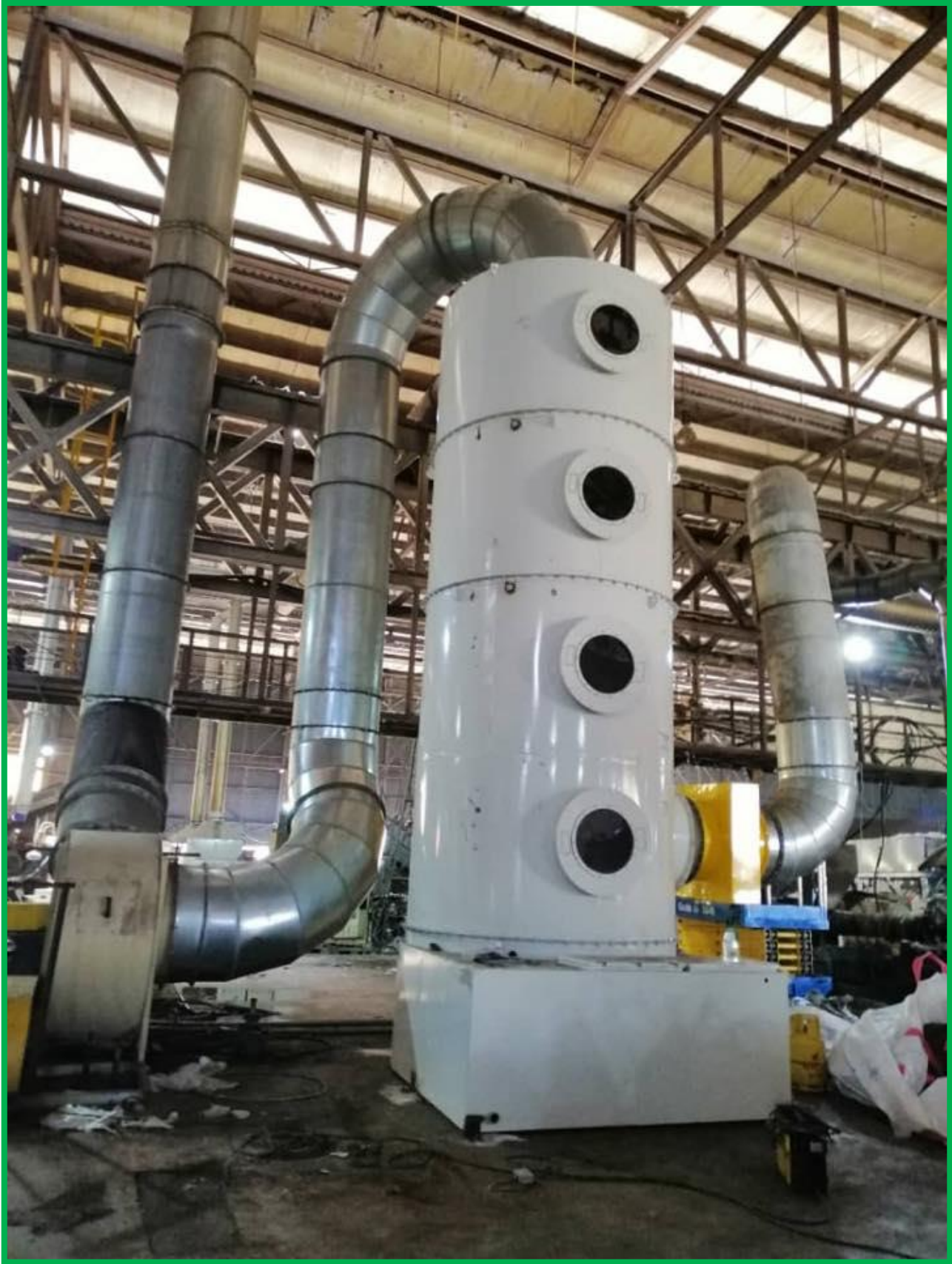
Scrubber System – Sungai Petani
