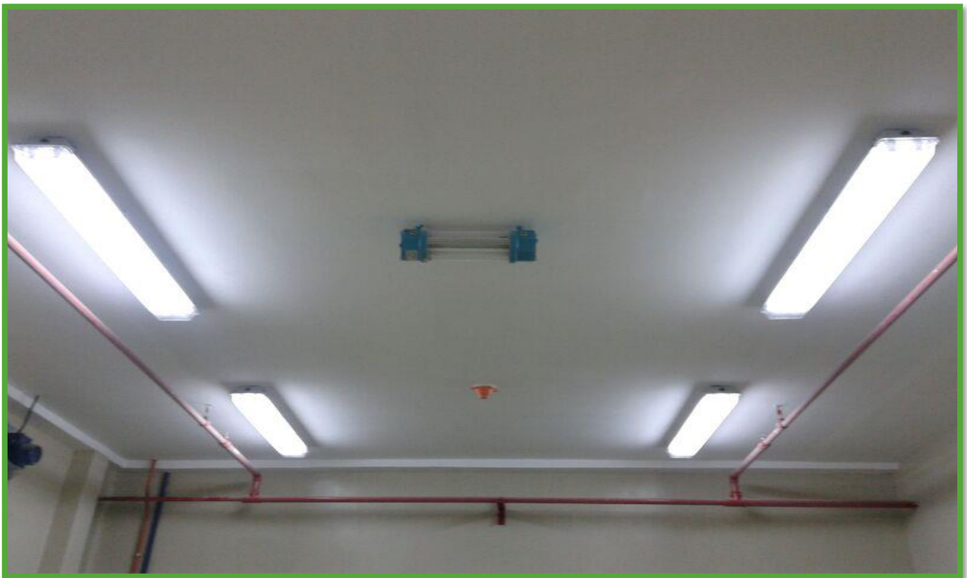
Fire Rated Ceiling – Prai
