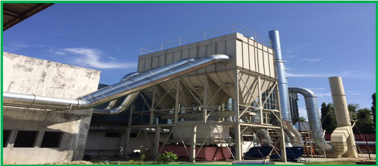
Mechanical Dust Collector System – Sungai Petani
