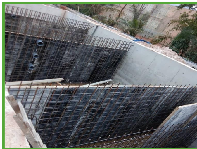
Waste Water Treatment Plant
