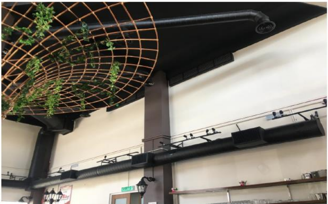
Air Cond Duct Work – Sungai Petani
