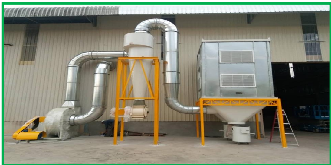
Filtration System – Jawi
