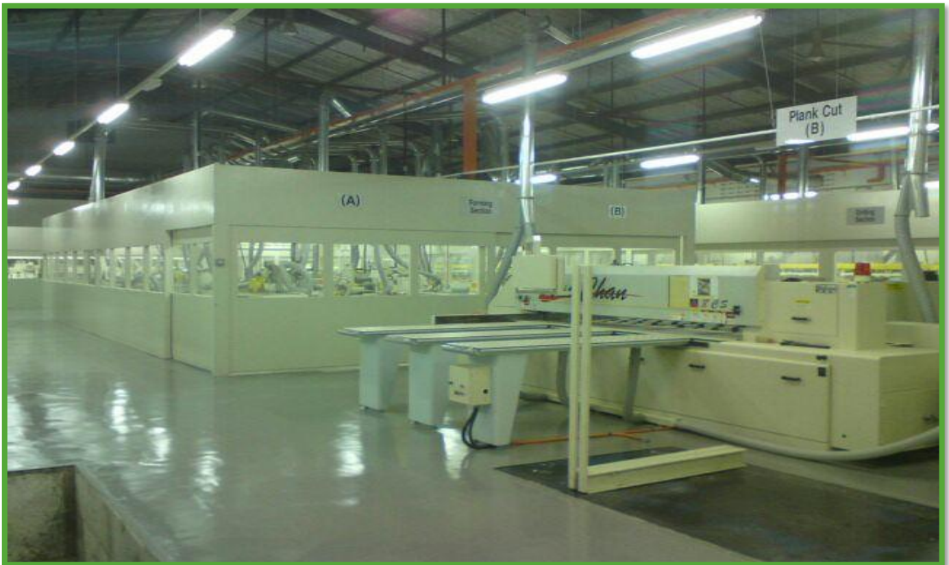
Plywood Sound Proof Machine Room – Prai
