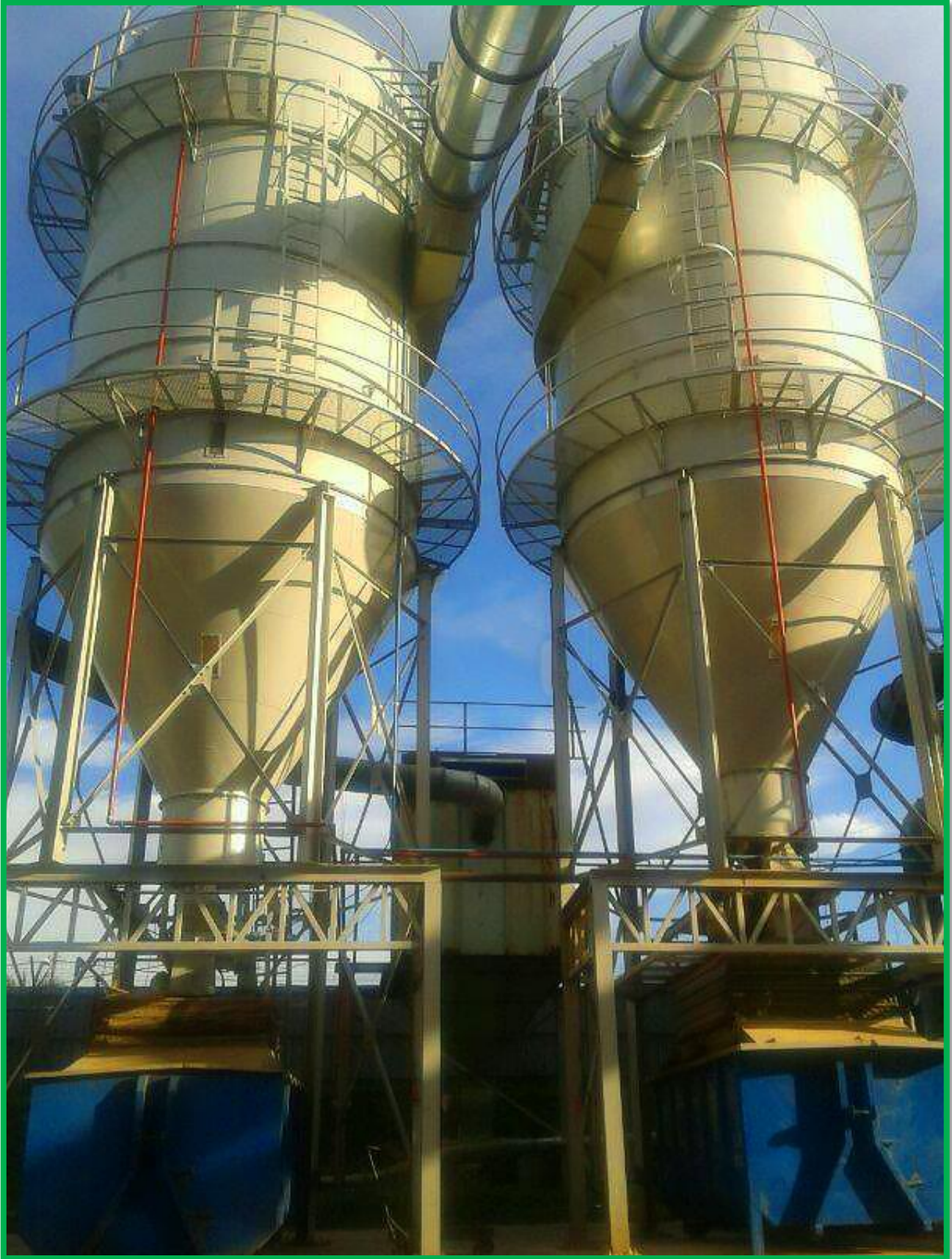
Mechanical Jet-Pulse Dust Collector System (Two-In-One) – Sungai Petani
