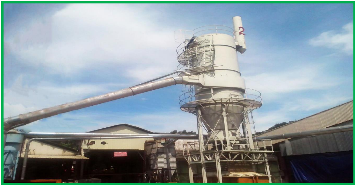
Mechanical Jet-Pulse Dust Collector System – Prai
